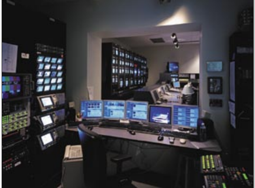
The tape/server operations room looks into the production room. It uses Sony Digital Betacam, a Grass Valley M-Series iVDR, and DNF and Lance controllers.
